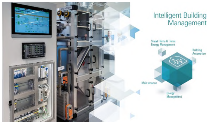
Exhibitors present pioneering innovations for tomorrow's buildings in the 'Intelligent building control' thematic category. Source: Messe Frankfurt Exhibition GmbH
